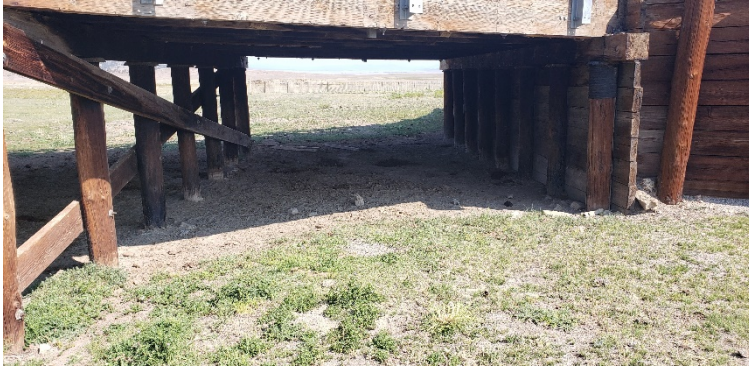
Photo 4. Wetland 1 , looking northwest under Bridge I-13-H where Wetland 1 narrows and stops under bridge and become a small scour pool in front of the abutment.
